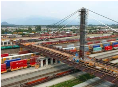
Temporary stay-cable systems for the launching stage were used for the first time in North America
