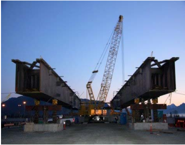
With an average weight of 85 tons each, 44 girders were used in the bridge construction
